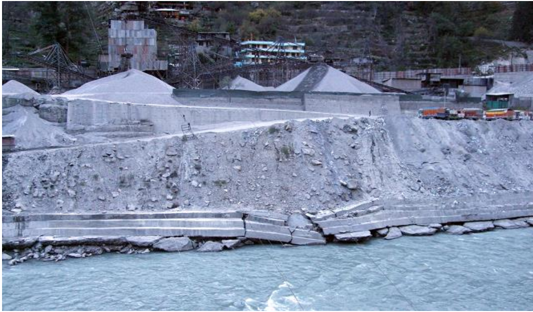
Fig.-5 Broken flood protection wall along the Sulej River downstream of Karcham Wangtoo dam, Photo taken on Nov 10 2010
