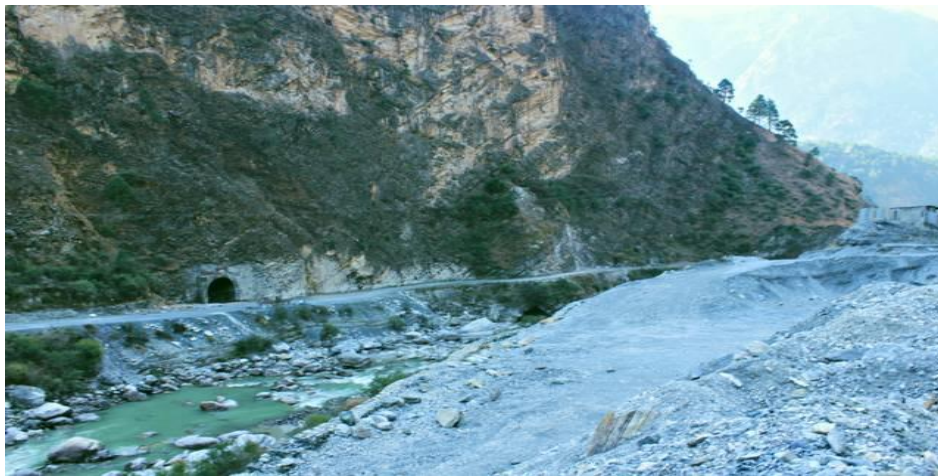
Fig-3 Muck Dumping along the Sainj River by Parvati Hydropower Project ( http://hillpost.in/2014/04/beas-a-dying-free-flow-himalayan-river-photo-essay/98678/ )
