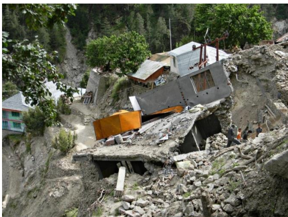
Fig.-6 Remnants of houses damaged by the landslide at Pangri village near Reckong Peo town ( http://www.epw.in/journal/2015/18/reports-states-web-exclusives/kinnaurs-curse.html )
