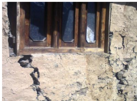
Fig.-7 Cracks developed in the houses of the native people ( Katoch, Anup et al, 'Impact of Nathpa Jhakri Hydroelectric Power Project on the Environment and Livelihood in Kinnaur and Shimla Districts of Himachal Pradesh, 2014, CSK HPKV Palampur H.P. )
